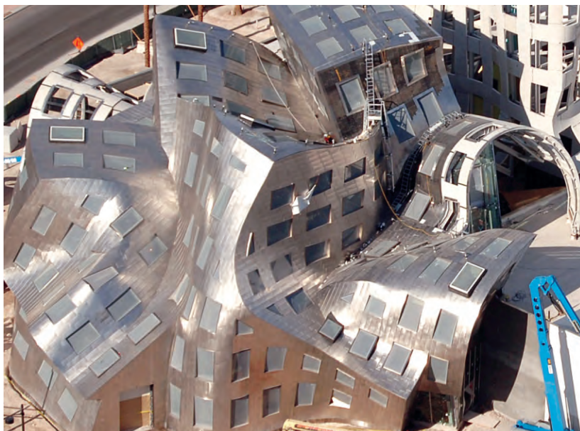
Cleveland Clinic Lou Ruvo Center for Brain Health, under construction, year end 2009
